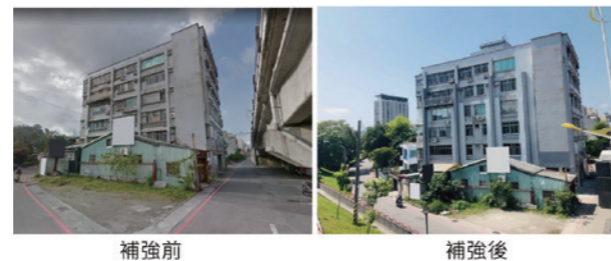
▲ 採用新增剪力牆、翼牆等工法進行耐震補強 Seismic retrofit by shear walls, wing walls, etc.
